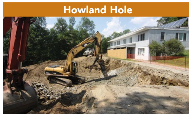
In July, excavation started for the new dormitory building to replace Howland, known by students as “New Howland.” No sign of Emily Mather’s grave yet (see page 15).
